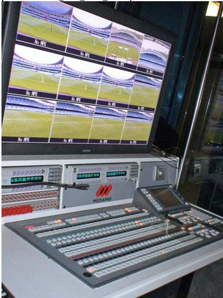
Inside – Systems from RTS
